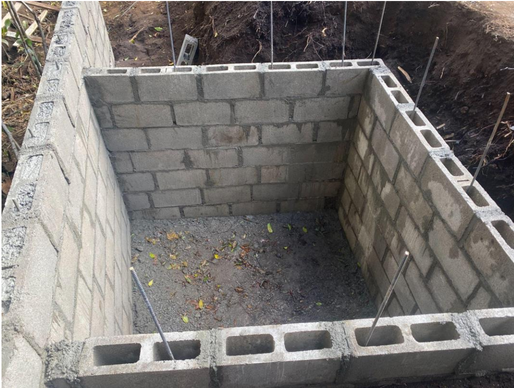
Inside of a septic tank
